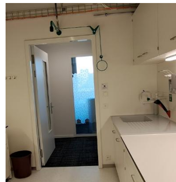
Emergency shower above the entrance door
