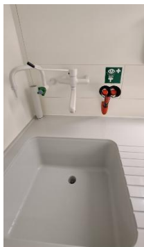
Eyewash station by the sink
